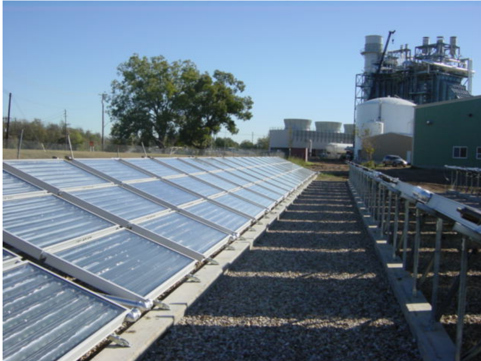
Figure 12: Austin Energy solar collector field for polygeneration (Courtesy: Solargenix).
