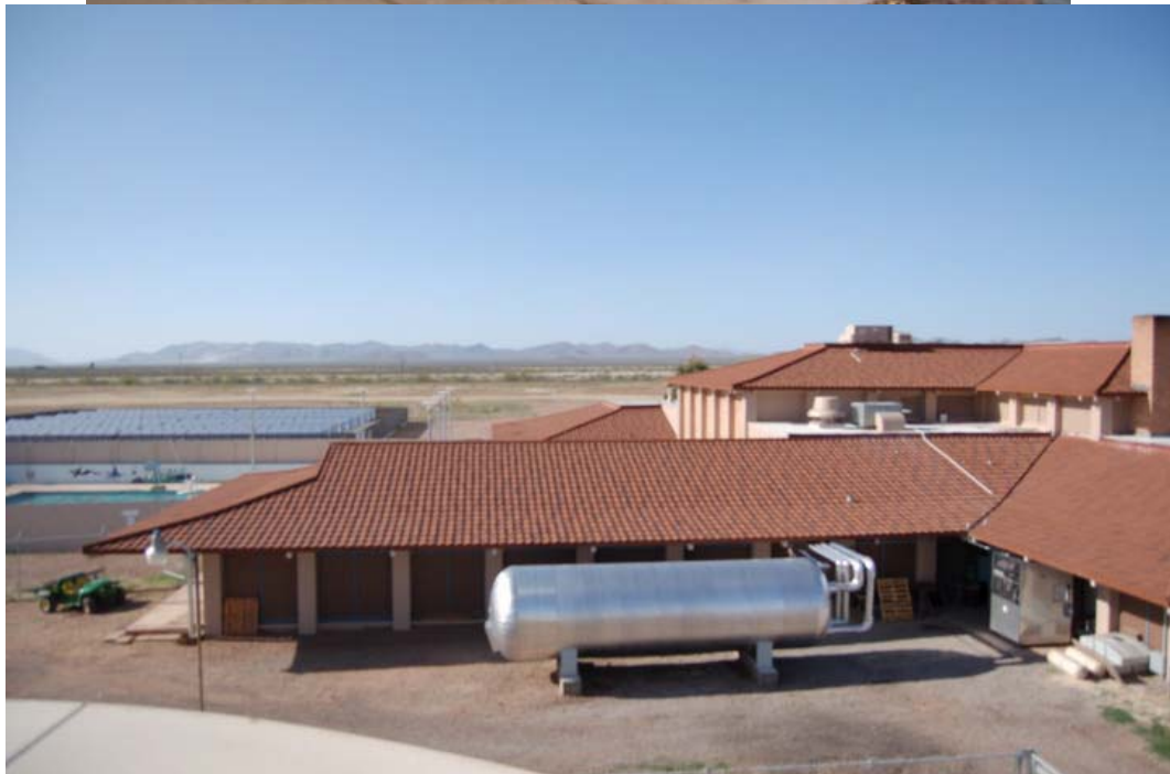
Figure 10: 60 ton solar-fired Helichiller (above) with storage tank (below) (Courtesy: Don Erickson, Energy Concepts).
